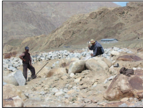
Stone contractors breaking stone near Domkhar. The rapid upsurge in construction has created a huge demand for stone. © Martin Vemier
